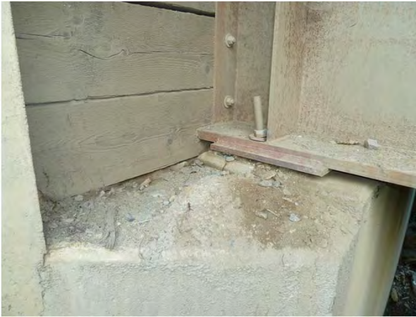
Figure 1-19: Bent anchor bolt woods end downstream side.
