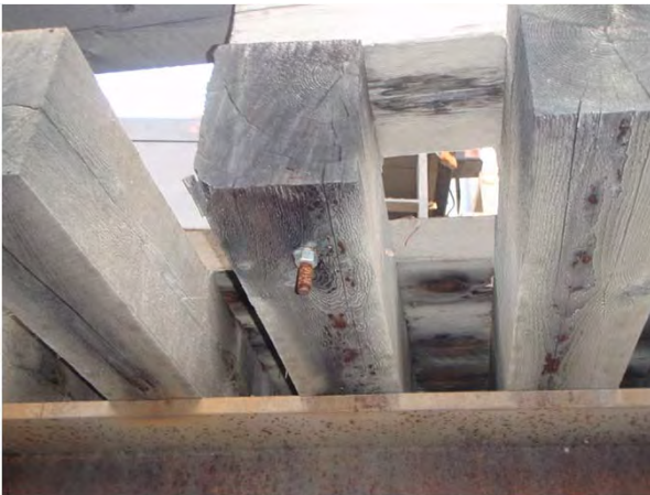
Figure 1-7: No malleable washer on underside of curb rail connection.
