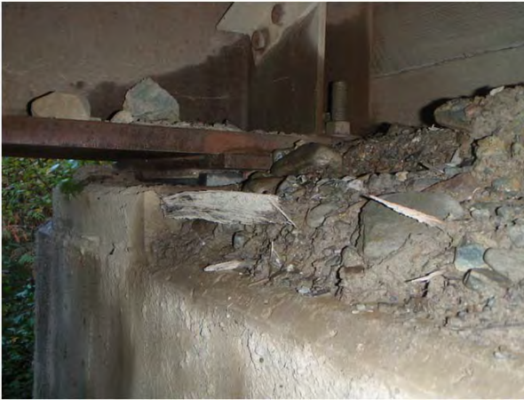
Figure 1-13: Camp end upstream bearing (note debris accumulation in bearing area.
